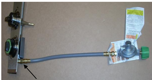
LP HOSE AND REGULATOR CONNECTION TO MANIFOLD
